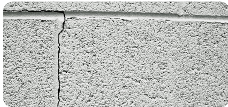
Exterior surfaces with plaster cracks upto 10mm
