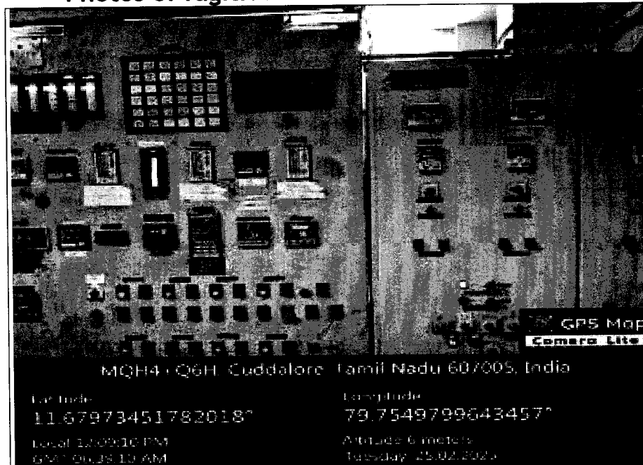
TPP Operation control 'PLC system
